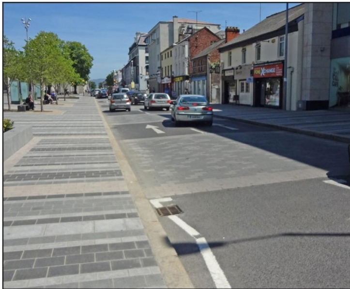
Figure 3.16: Illustration of surface treatments in Dundalk, Co. Louth. These treatments enhance the sense of place by expanding the square into the adjacent streets and are an effective way of improving pedestrian mobility and calming traffic.
